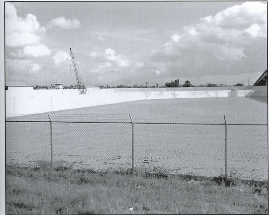
Cousins Canal Walls Destrehan Bridge to Sector Gate Harvey Canal, Jefferson Parish, Louisiana
