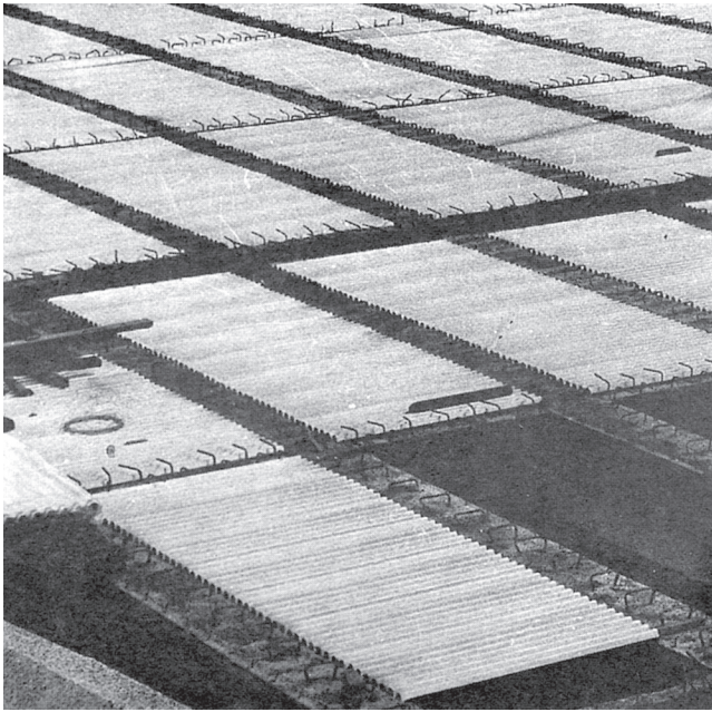
Fig 5.9 — Stay-in-place corrugated metal forms are supported on precast concrete girders. Nails cast in the girders are bent over to hold the form in place.
