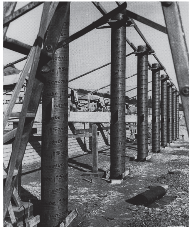
Fig. 5.7 — Fiber tube column forms require bracing to keep them plumb and a template at the base for accurate positioning.
