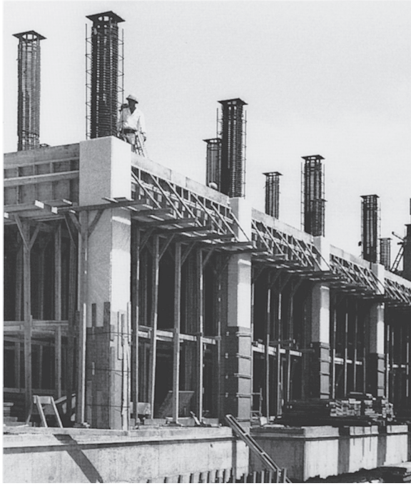
Fig. 5.11 — Precast concrete panels served as column forms, thus creating an architectural surface. During construction, the bases of the columns were protected with wood sheathing held in place with metal straps.
