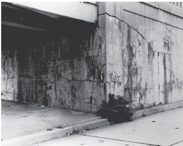
Fig. 3.8.1—Cracking caused by abnormal expansion due to alkali-silica reaction.
