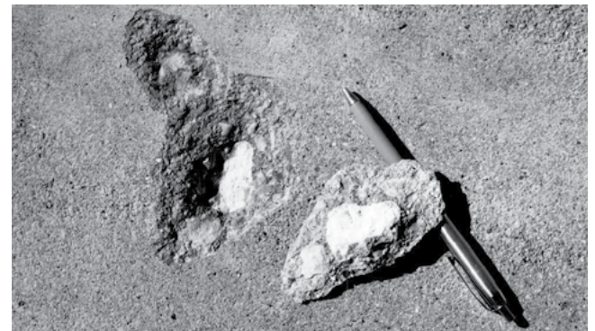
Fig. 3.7.3—Popout due to unsound aggregate particles.
