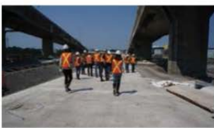
Students walking on the new Turcot interchange while the old structure (left and right) is still in use
