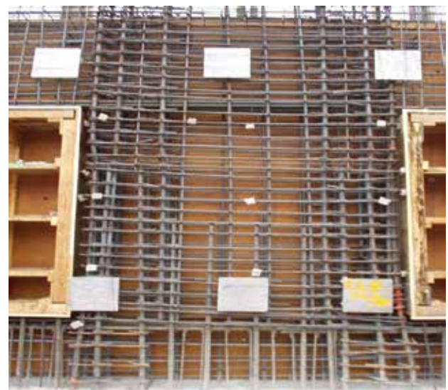
Fig. 5: A reinforced concrete wall with embeds and penetrations, shown prior to closure of the formwork. The embeds adjacent to the wall penetrations interfere with the vertical bars in the wall (photo courtesy of Bruce Suprenant)
