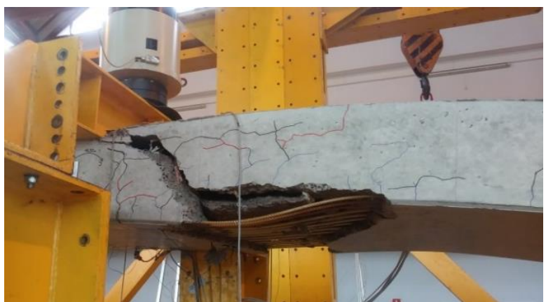
Crack after concrete cover failure
