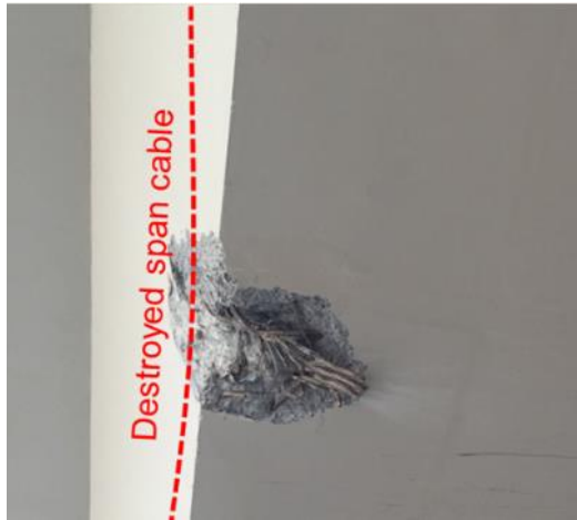
Damage of the existing structure
