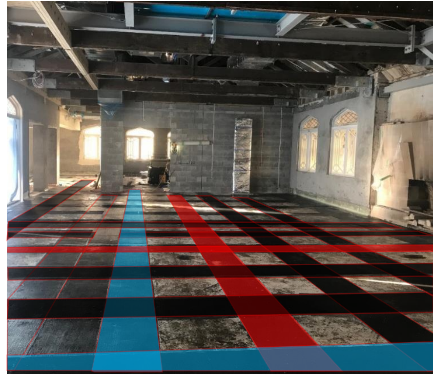
(b) Concrete diaphragms strengthened by FRP
