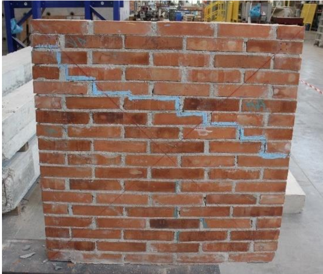
Stair-stepped crack (sliding phenomenon)
