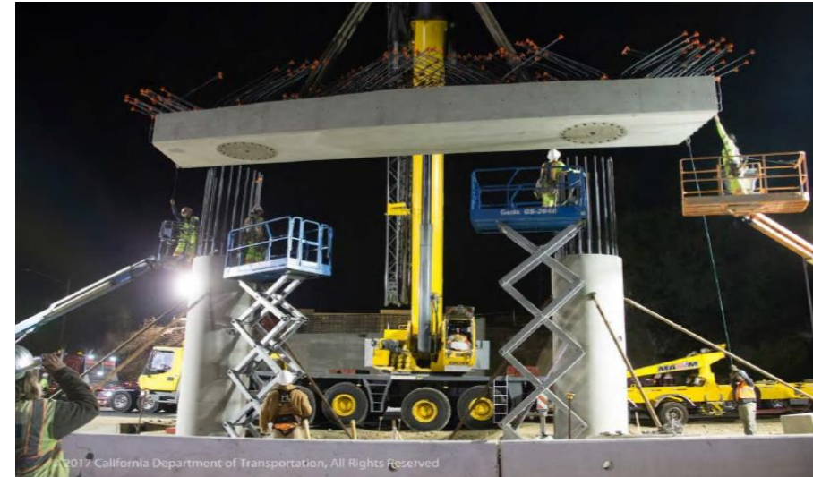
Precast columns and drop bent cap for Laurel Street Overcrossing project in CA (courtesy of Dorie Mellon)
