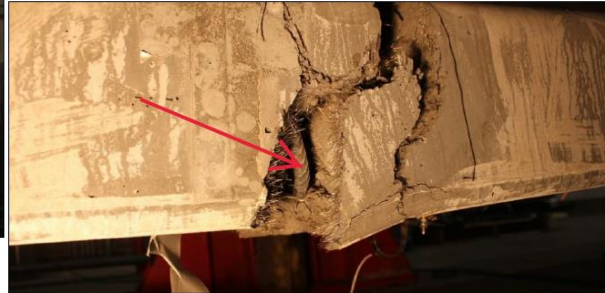
Close view of failure location showing stirrup
