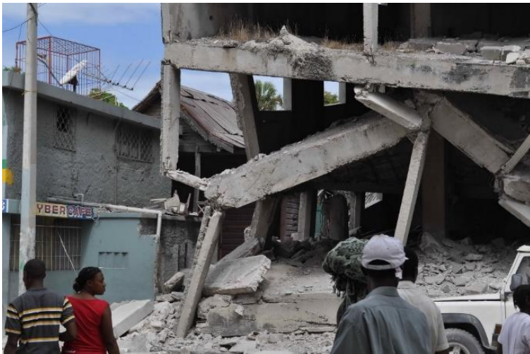
Collapse of second and third floor concrete column by earthquake
