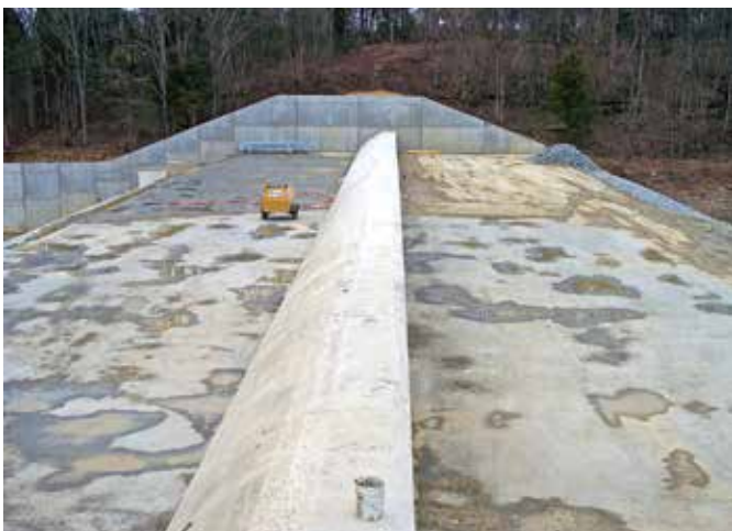
Fig. 10: Fox Creek Dam, Fleming County, KY, is an example of an ogee weir cast over RCC (© photo courtesy of Schnabel Engineering)
