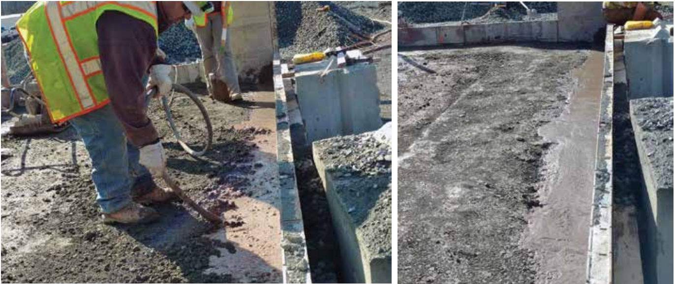
Fig. 6: A grout-enriched facing mixture is placed between previously placed RCC and formwork: (a) a mechanical vibrator is used to consolidate and combine the two mixtures; and (b) a completed test section (© photos courtesy of Schnabel Engineering)
