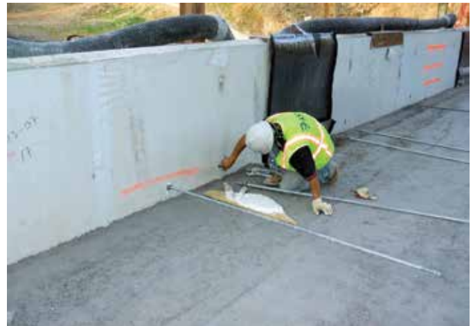
Fig. 7: Facing panel installation with anchors embedded between RCC lifts (© photo courtesy of Schnabel Engineering)
