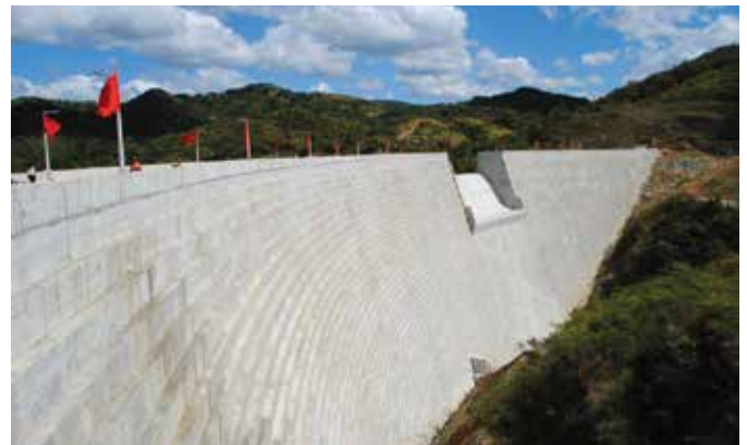
Fig. 4: The RCC arch-gravity Portugués Dam has a total length of 1230 ft (375 m) (photo courtesy of U.S. Army Corps of Engineers)
