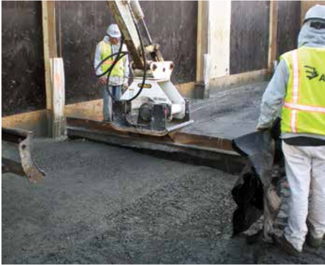
Fig. 11: Transverse joint construction by inserting and removing a plate in fresh RCC (© photo courtesy of Schnabel Engineering)
