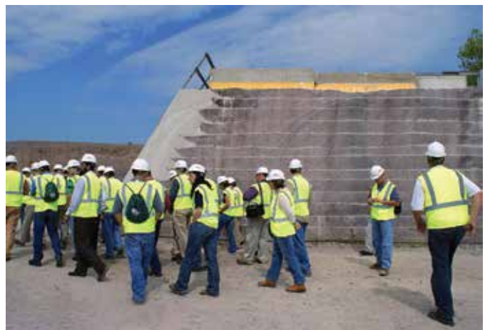
Fig. 8: A test section is used to demonstrate conventional concrete facing for Taum Sauk Dam (photo courtesy of ASI Construction LLC)
