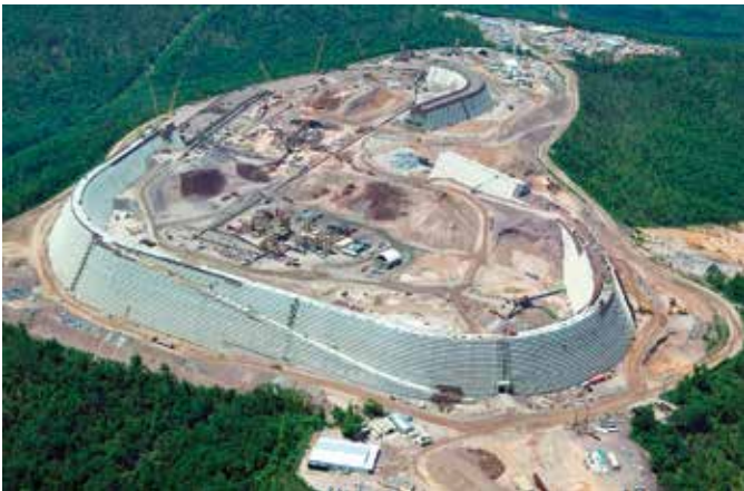
Fig. 2: Taum Sauk Dam, designed by Paul C. Rizzo Associates, Inc., is composed of several million yd 3 of RCC and with inner and outer facings of conventional concrete (photo courtesy of ASI Construction LLC)
