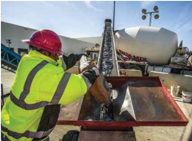
Before each concrete truck entered the building, steel fibers were added at a dosage of 23 lb/yd 3 (13.6 kg/m 3 ) (photo courtesy of Jon Humphrey)
