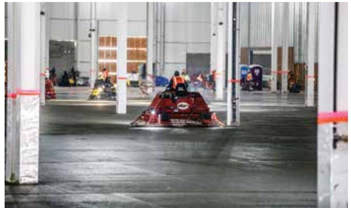
The operators of 38 ride-on trowels made sure that the finished floor had high FF/FL numbers—achieved values were 56/42 (photo courtesy of Jon Humphrey)
