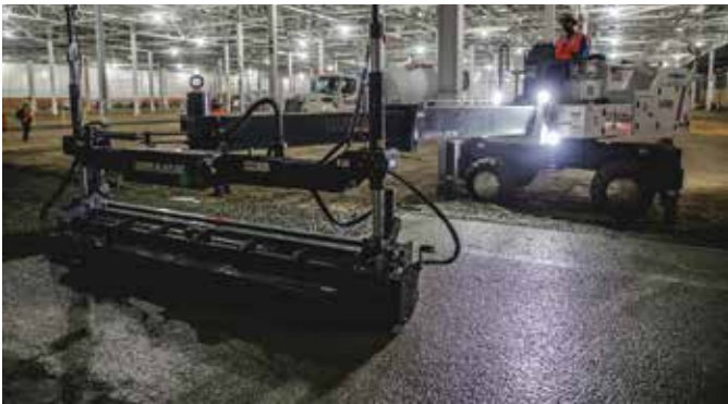
Four laser screeds were used during the placement, helping to provide a slab surface that was within 3/16 in. (5 mm) of plane over the huge floor area (photo courtesy of Jon Humphrey)
