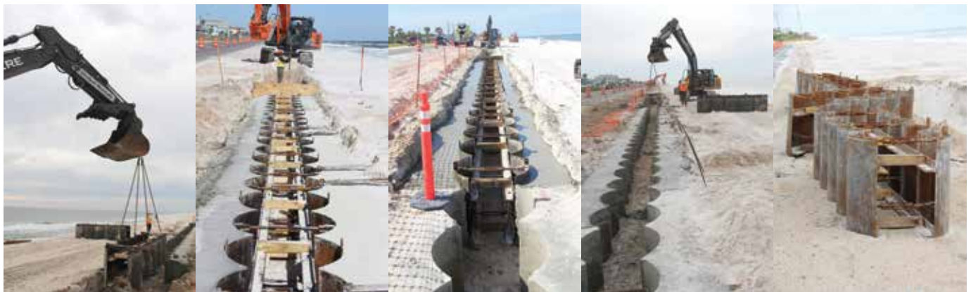
Fig. 4: Construction of the guide wall, a concrete template that was used to align and locate the seawall’s secant piles and provide positional restraint and the required verticality of the piles. The guide wall was removed prior to construction of the pile cap
