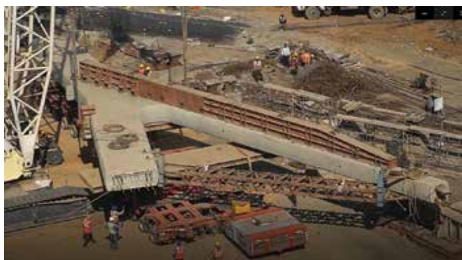
Fig. 8: A precast column is transported to the erection point using trailers. The long, slender legs of precast column units required strongbacks and braces for erection
