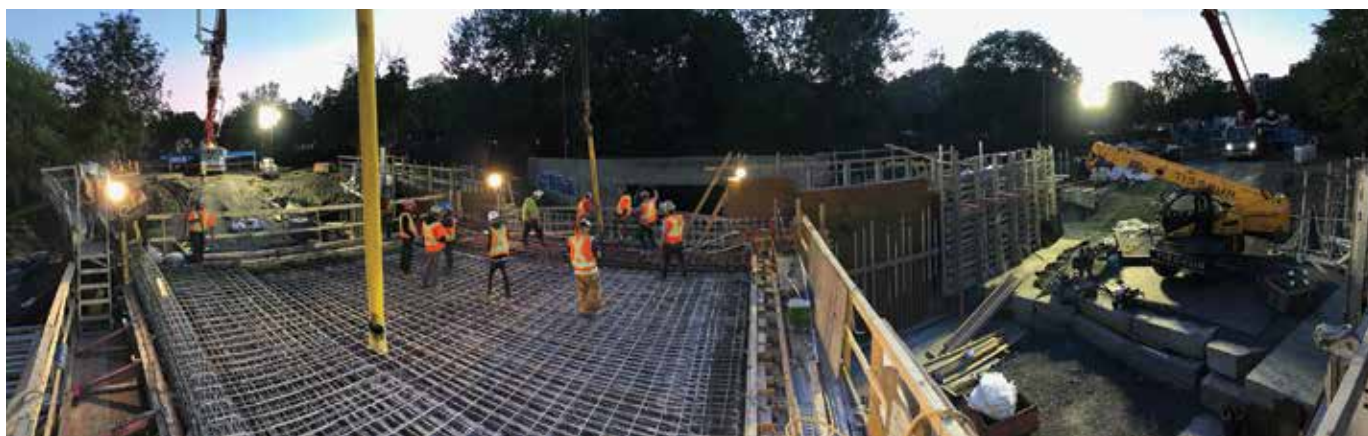
Fig. 12: One of two bridges under construction in Montréal comprising concrete with 10% cement replacement with Type GS GGP. The bridges will be instrumented and closely monitored by the University of Sherbrooke and the Ville de Montréal (photo courtesy of Ville de Montréal)
