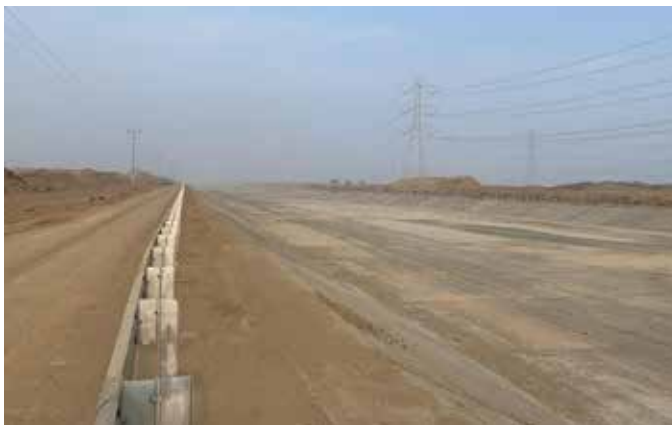
The finished reinforced concrete channel in Jizan will direct flood water away from roads and industrial production facilities (photo courtesy of Al Yamama Group)
