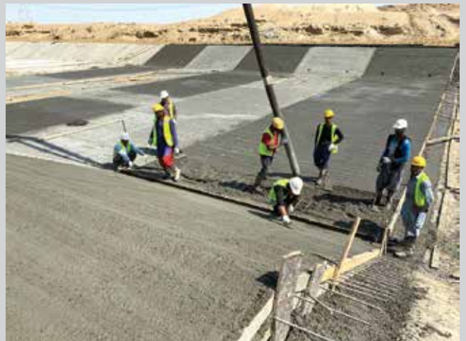
Step 6: Concrete is placed on top of the reinforcing bars, then tamped and consolidated
