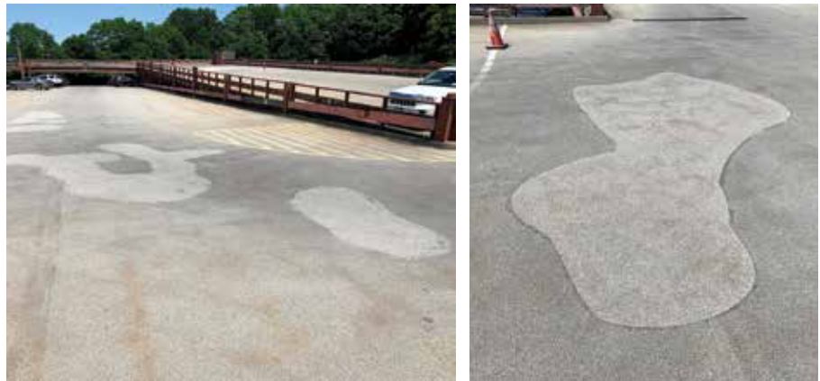
Fig. 7: A parking garage deck in Utica, NY, USA, repaired with the rubber-modified repair material, after 4 years in service
