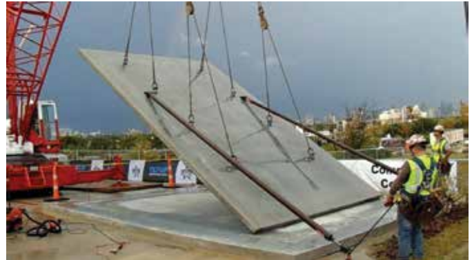
Fig. 3: A 4.5 in. (114 mm) thick tilt-up concrete panel designed using performance-based design principles is lifted (from Reference 16)
