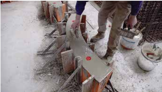
The window frames near completion. After the joints were mortared, the frames were painted to complete the façade restoration
