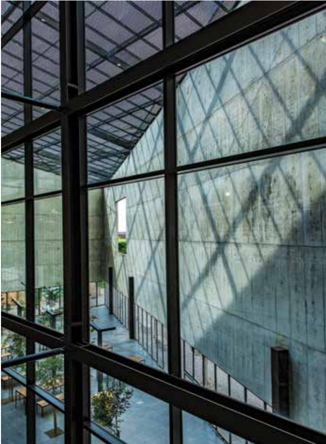
Fig. 3: Exterior walls are supported by steel columns cast in footings and sitting on the inside of the wall
