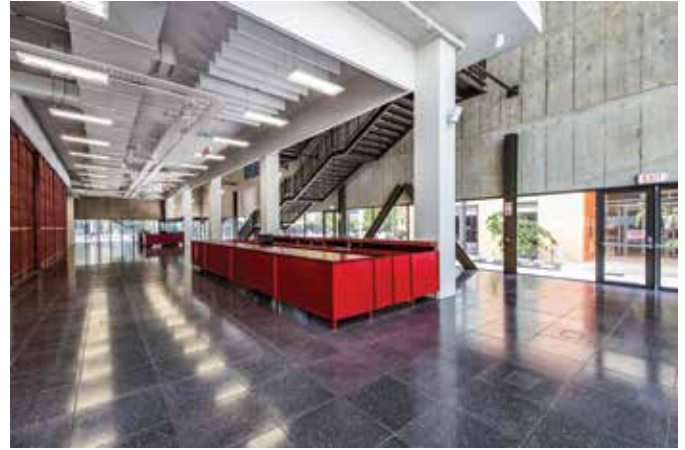
Fig. 4: Steel A-frames of the ground floor auditorium provide additional support for the structure
