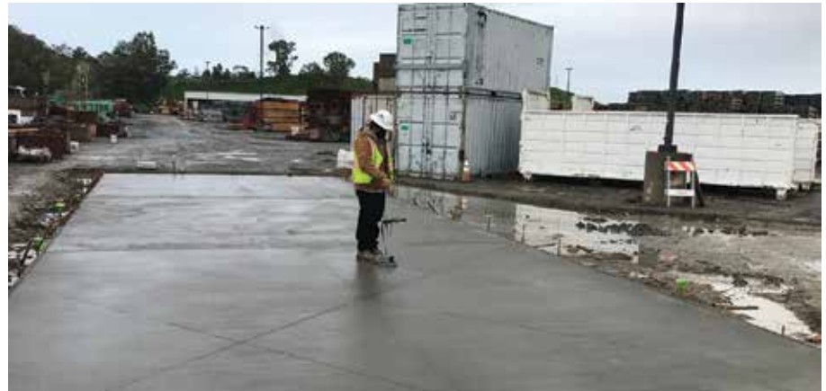
Fig. 7: Technician uses a Dipstick® to measure F-numbers on parallel measurement lines for each test panel section: swirl, broom, pan float, and bullfloat finish
