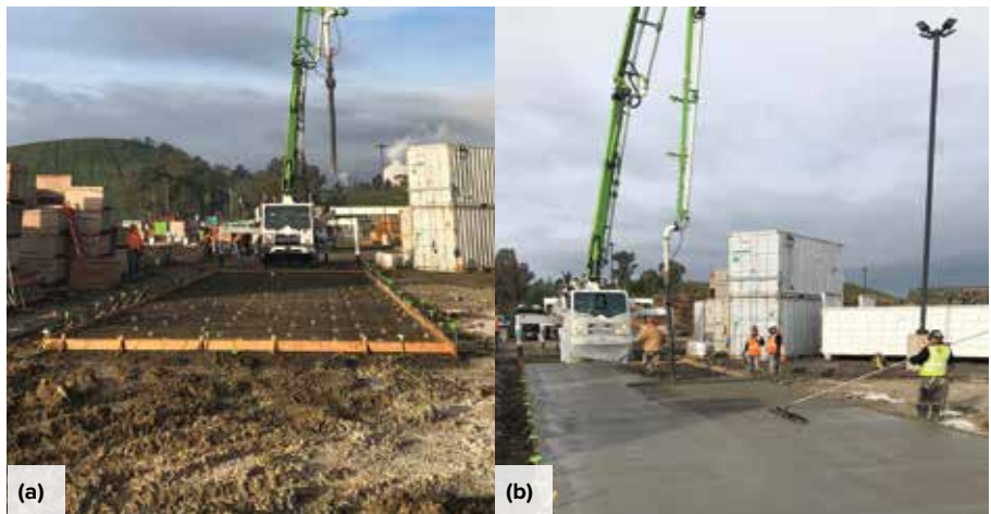
Fig. 4: Initial steps in the construction of a 20 x 80 ft (6 x 24 m), 6 in. (150 mm) thick test panel used to evaluate the effects of swirl and broom finishes on F-numbers: (a) formwork, reinforcement, pump, and crew are in place; and (b) concrete placement nears completion. Concrete was pumped, internally vibrated, struck off using a 16 ft (5 m) long screed, and smoothed using a 6 ft (2 m) channel float
