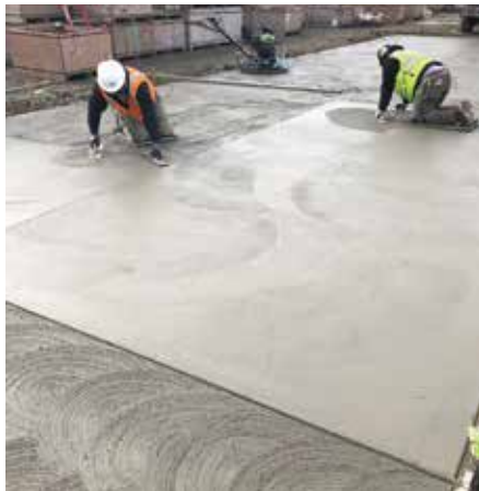
Fig. 6: For a broom finish, after panning, finishers on kneeboards used a hand float and trowel to prepare the surface for brooming. The swirl finish was placed on the panned surface
