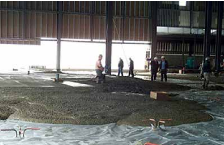
Fig. 3: An SFRC slab-on-piles designed using the Belgian method (Montréal-Mirabel, 2001). Concrete was placed by direct discharge of concrete trucks. The piles are on a 4 x 4 m (13 x 13 ft) pile grid (four bent reinforcing bars can be seen at each pile)
