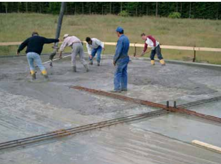
Fig. 4: An SFRC elevated slab constructed with flowable concrete. Designed according to method described in the ACI 544.6R-15 report, this slab includes integrity reinforcement—bottom reinforcing bars extending from column to column—to prevent progressive collapse in the event of overload or damage
