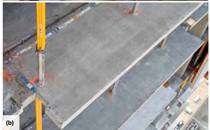
Fig. 3: Structural thermal breaks in balconies: (a) during placement of balcony concrete; and (b) after placement of balcony and slab concrete. Note: Modules are installed with the top plate flush with the exterior concrete structure. The white bars are GFRP bars
