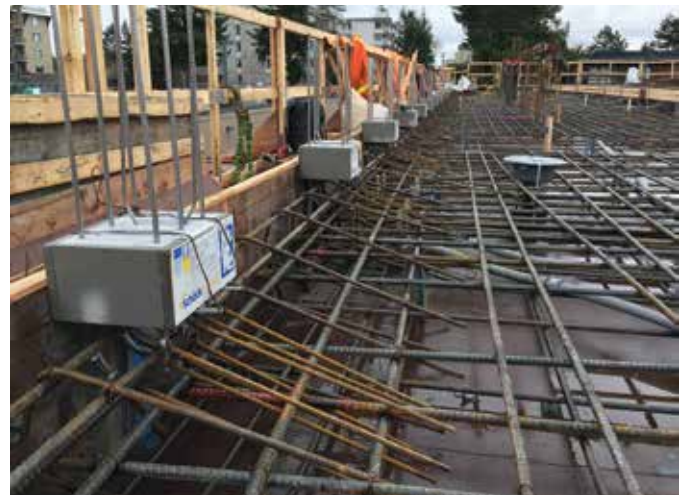
Fig. 4: Thermal breaks for parapets are installed at the vertical wooden parapet forms and tied into the horizontal reinforcing bars. Reinforcing bars are fabricated to transfer both bending and shear across the insulation layer
