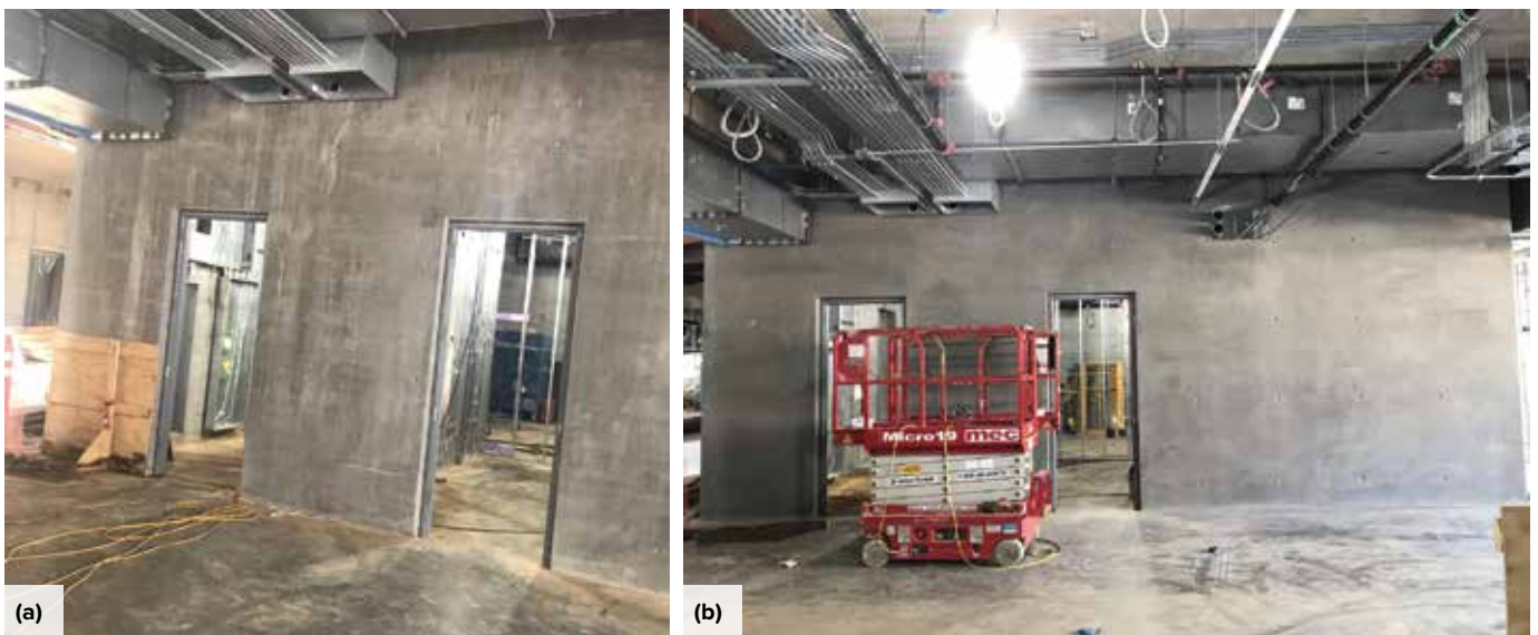
Fig. 3: A shear wall: (a) the surface initially exhibited efflorescence and laitance; and (b) the same surface after cleaning
