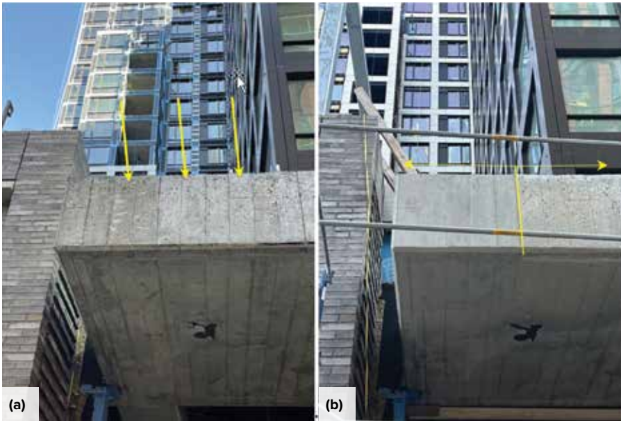
Fig. 4: A structural canopy: (a) the vertical surface initially exhibited numerous bugholes; and (b) a progress photo shows the benefits of patching and cleaning to improve uniformity
