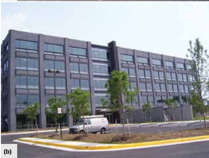
Fig. 6: A building with precast concrete façade elements: (a) during construction, efflorescence concealed the beauty of the elements; and (b) a final cleaning resulted in improved color and uniformity
