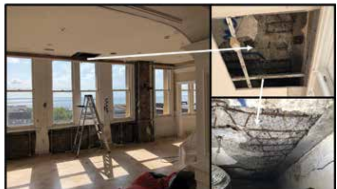
Fig. 4: Corrosion of an interior slab in an historic building constructed circa 1910-1911
