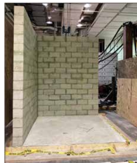
Fig. 3: CMU wall construction completion (photo courtesy of CEIST Lab at University of Colorado Boulder)
