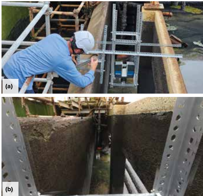
Fig. 6: Using lidar scanning to capture the condition of an inaccessible area: (a) mounting; and (b) an output
