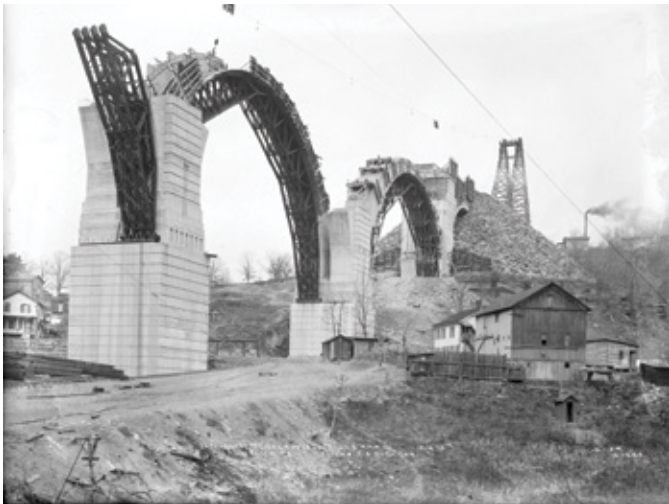
Steel formwork for the arches begins to take shape in December 1913 (photo courtesy of the Steamtown National Historic Site Archives)
