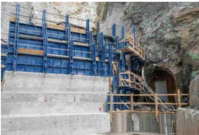
Doka custom steel formwork for RCC used in the Gross Reservoir expansion project (©Doka)
