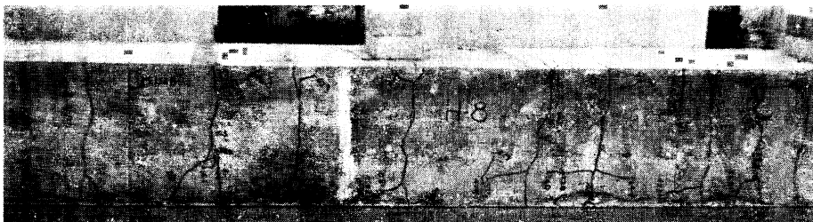
Fig. 4—With two #11 bars at approximately same stress as in Fig. 3, longitudinal cracking is much reduced, although still obvious
