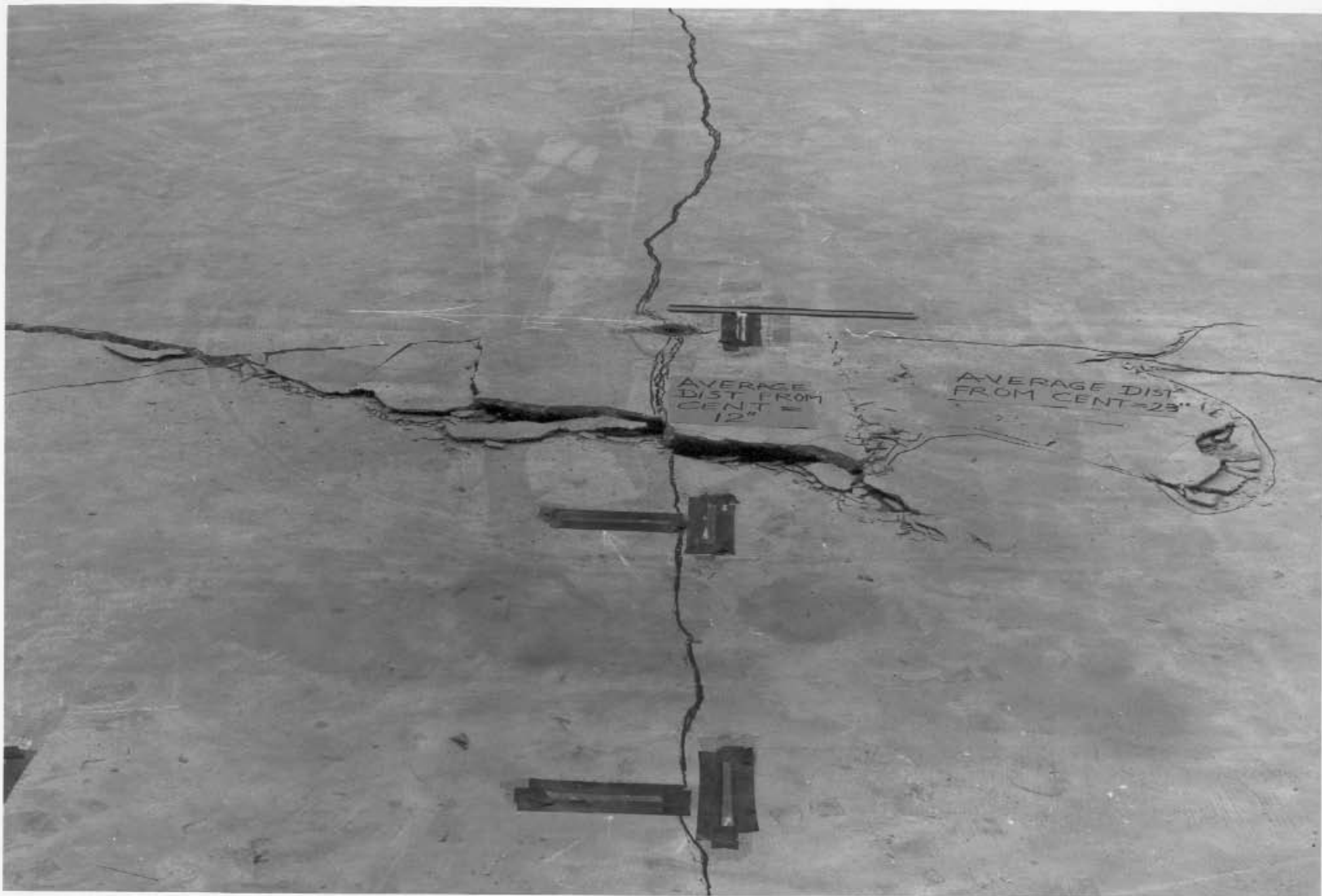
PHOTOGRAPH 8: CENTER SUPPORT AFTER FAILURE
