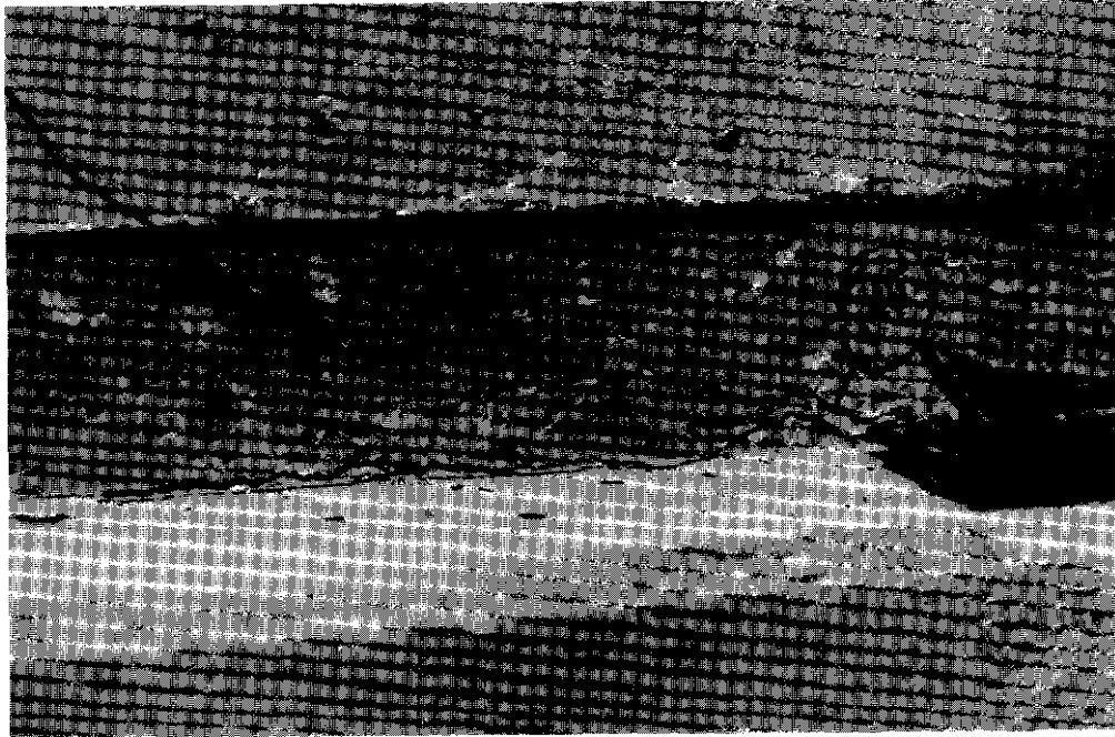
Fig.4.7 - Crack at ledge/web junction - Specimen 1
