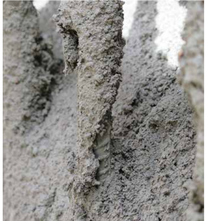
Fig. 3: Poor coating on the surface of reinforcing bar resulting from use of a mixture with inadequate rheology
