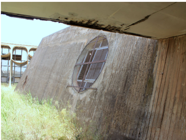
Fig. 2 The right side protected part, the left side exposed part.
