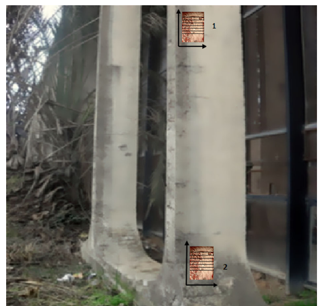
Fig. 4 The right side protected part, the left side exposed part of the straight wall.
