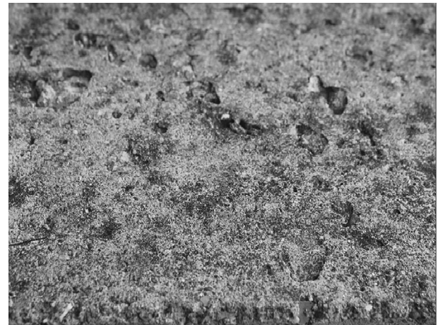
Fig. 14 The detachment of grain of various sizes on the exposed concrete surface.
