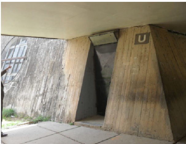
Fig. 1 Inclined wall intensely eroded.
