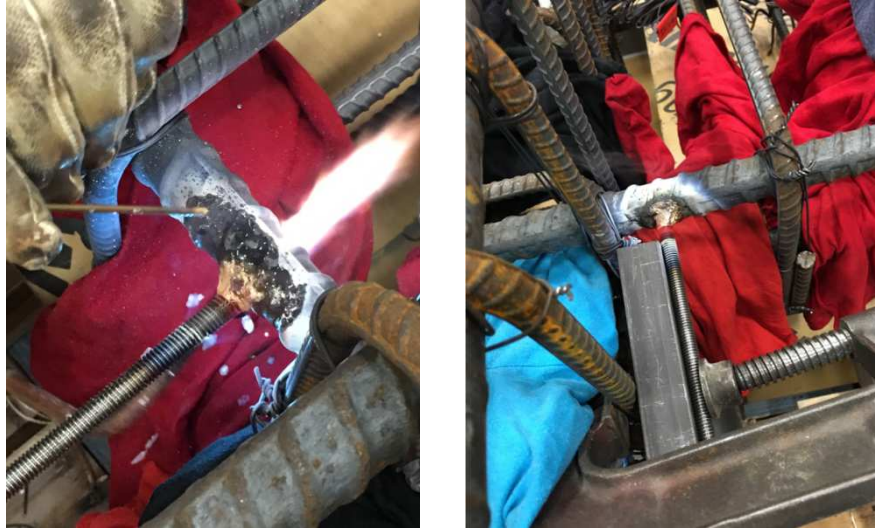
Figure A-17: Brass-Brazing Procedure - Step 5: Removal of Heat and Formation of Bond
