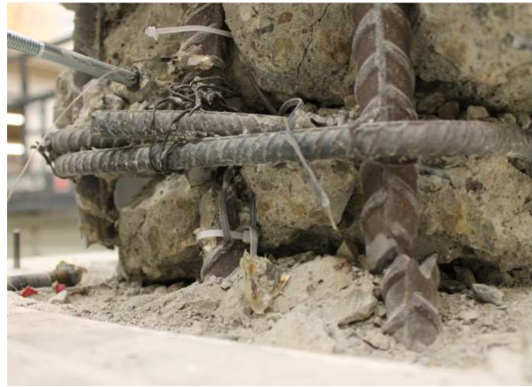
Figure 3.3.3: Failure Mechanism of SBL100 by Fracture of Longitudinal Bars
