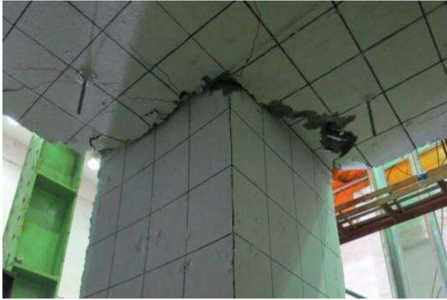
Fig. 4.25 – Slab Bottom Surface of Specimen G2 Near the Connection at Failure
