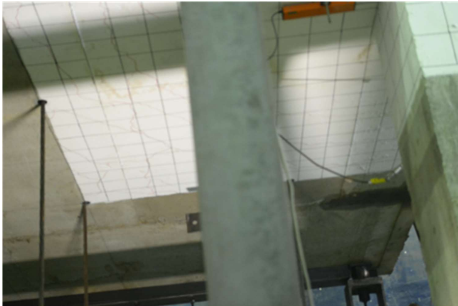
Fig. 4.14 –Slab Bottom Surface Crack Pattern of Specimen G1 at Initial Target Connection Shear.
