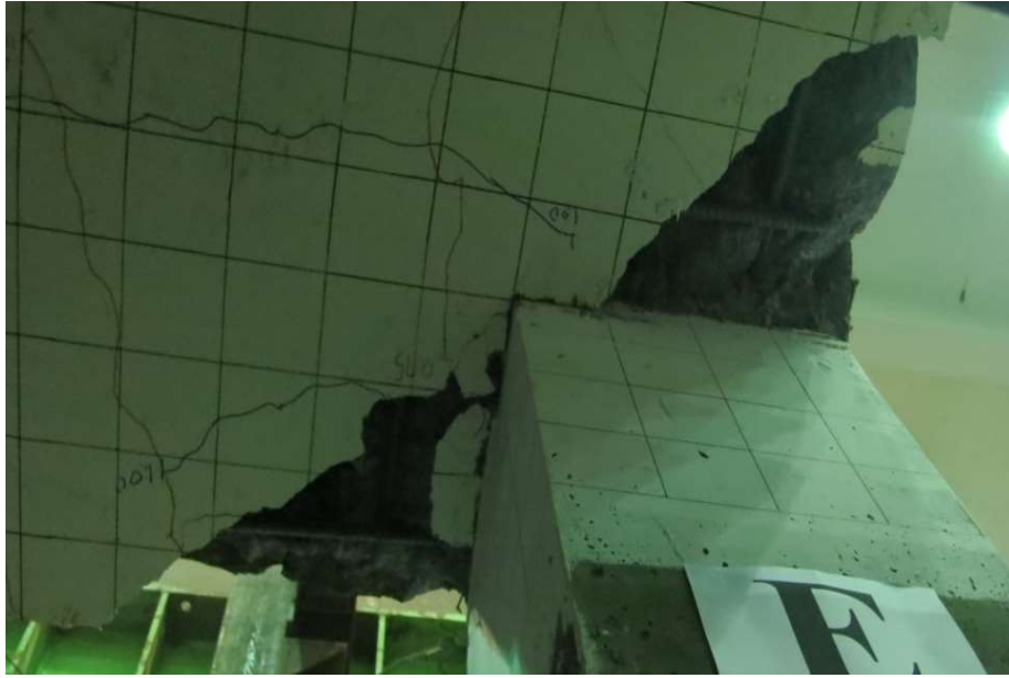
Fig. 4.47 – Slab Bottom Surface of Specimen R2 Near the Connection at Failure
