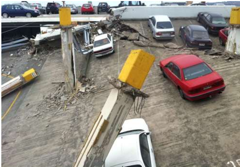
Fig.1.2 – Punching Shear Failure
