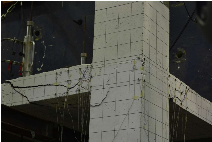
Fig. 4.37 – Crack Pattern on the North and West Slab Faces of Specimen R1 at 2.00% Drift
