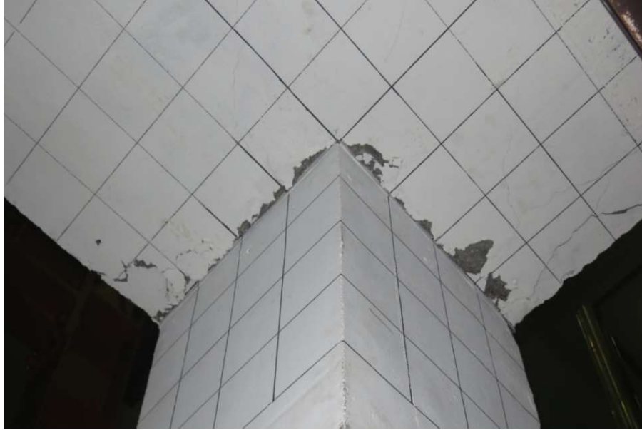
Fig. 4.32 – Slab Bottom Surface of Specimen G3 Near the Connection at Failure
