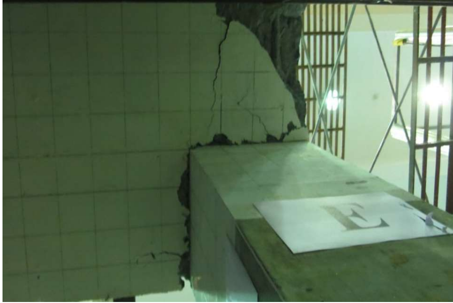
Fig. 4.55 – Slab Bottom Surface of Specimen R3 Near the Connection at Failure
