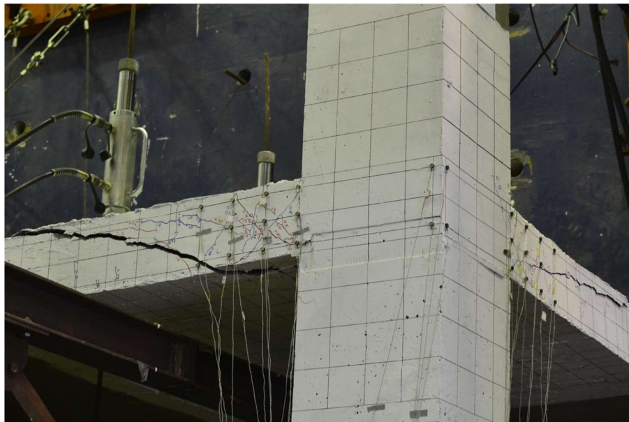
Fig. 4.43 – Crack Pattern on the North and West Slab Faces of Specimen R2 at 1.25% Drift
