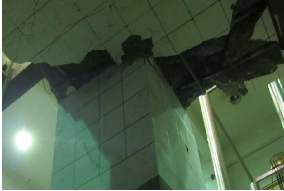
Fig. 4.41 – Slab Bottom Surface of Specimen R1 Near the Connection at Failure
