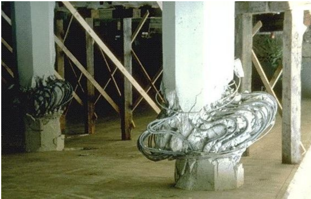
Figure 2-1 Reinforced concrete column crushing
