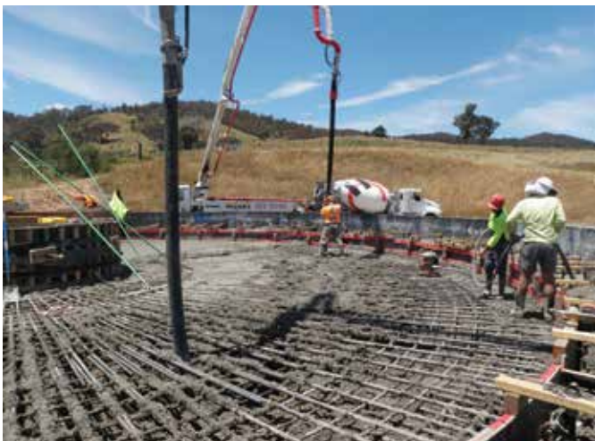
Fig. 1: Concrete placement of the antenna roof slab. Note that the concrete vibrator is not being applied near either delivery point
