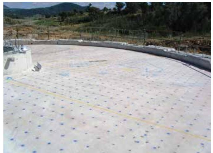
Fig. 2: Test grid marked on roof slab topside (blue lines outline underside concrete removal areas)
