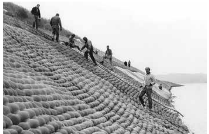
Fig. 1: A revetment (Fabriform® Filterpoint) is installed in 1967 on the Allegheny Reservoir, New York (photo courtesy of Construction Techniques, Inc.)
