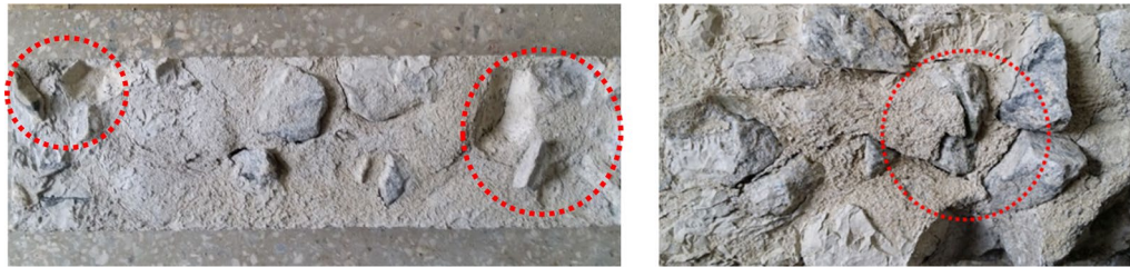
Fig. 3 Interfacial failure between recycled ballast aggregates and mortar in freezing–thawing tests (Yoo et al. 2016).
