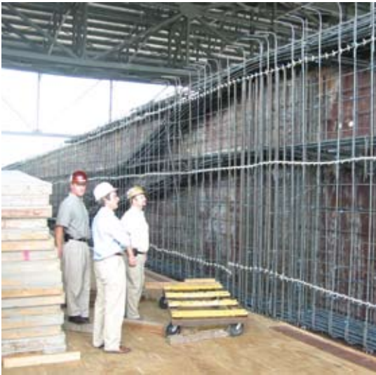
Fig. 2: Inspection of the tendons and reinforcement for a typical long-span girder (photo courtesy of Lawrence Kahn, Professor, Georgia Tech)
