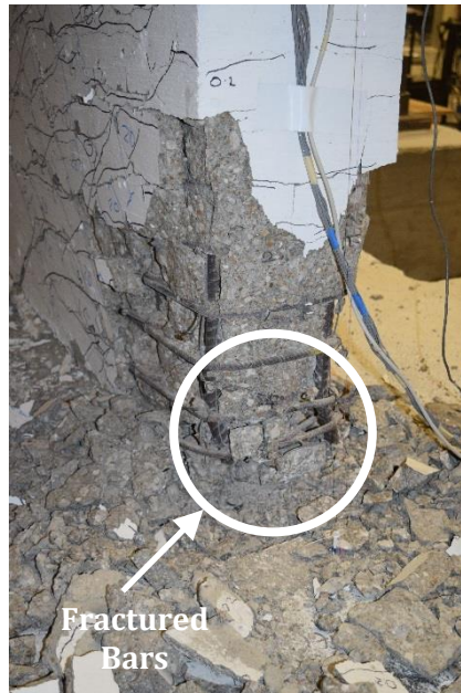
Figure 79 – Wall T4 with bar fracture in confined stem during second cycle to 4% drift ratio (stem in tension)
