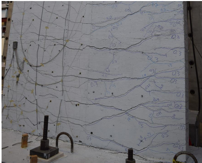
Figure 67 – Wall T4 without bar buckling or fracture in unconfined flange during second cycle to 2% drift ratio (stem in compression)
