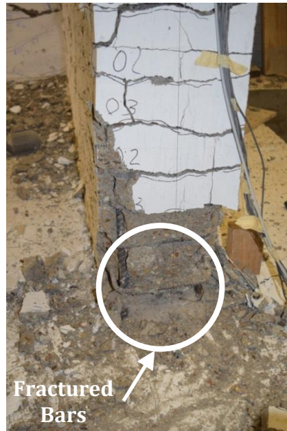
Figure 73 – Wall T1 with bar fracture in confined stem during first cycle to 4% drift ratio (stem in tension)
