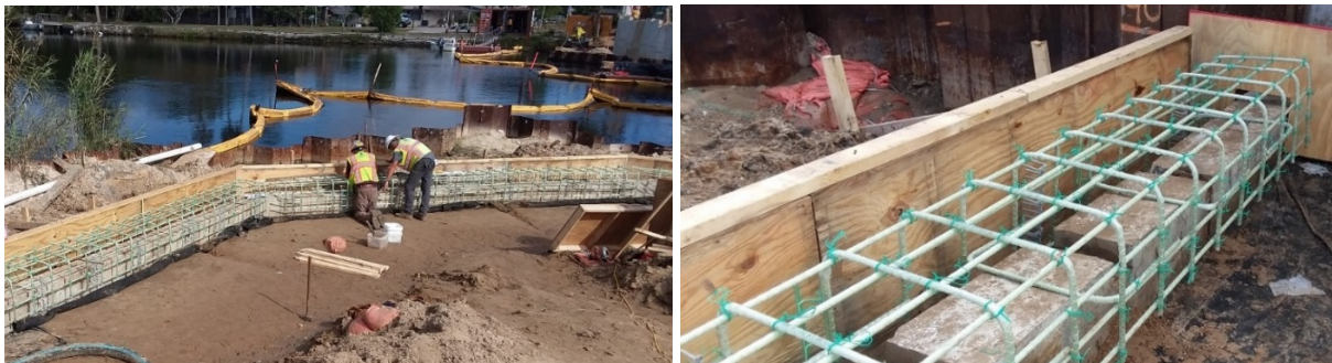
Figure 13 – GFRP bulkhead cap cage
