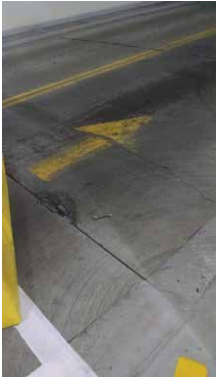
Fig. 3: Speed ramp cracks and damage in Structure B (Note: This photograph shows a different section of the speed ramp than the ultimate failure location, but the condition depicted is illustrative.)
