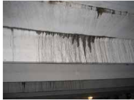
Fig. 2: Water stains on a cracked flange in Structure B
