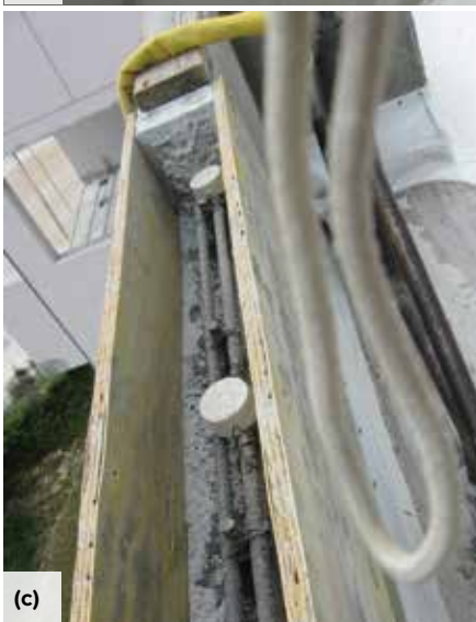
Fig. 5: In-progress repairs: (a) exposed reinforcement in corridor; (b) exposed reinforcement in parapet; and (c) GCP and formwork installed at parapet repair
