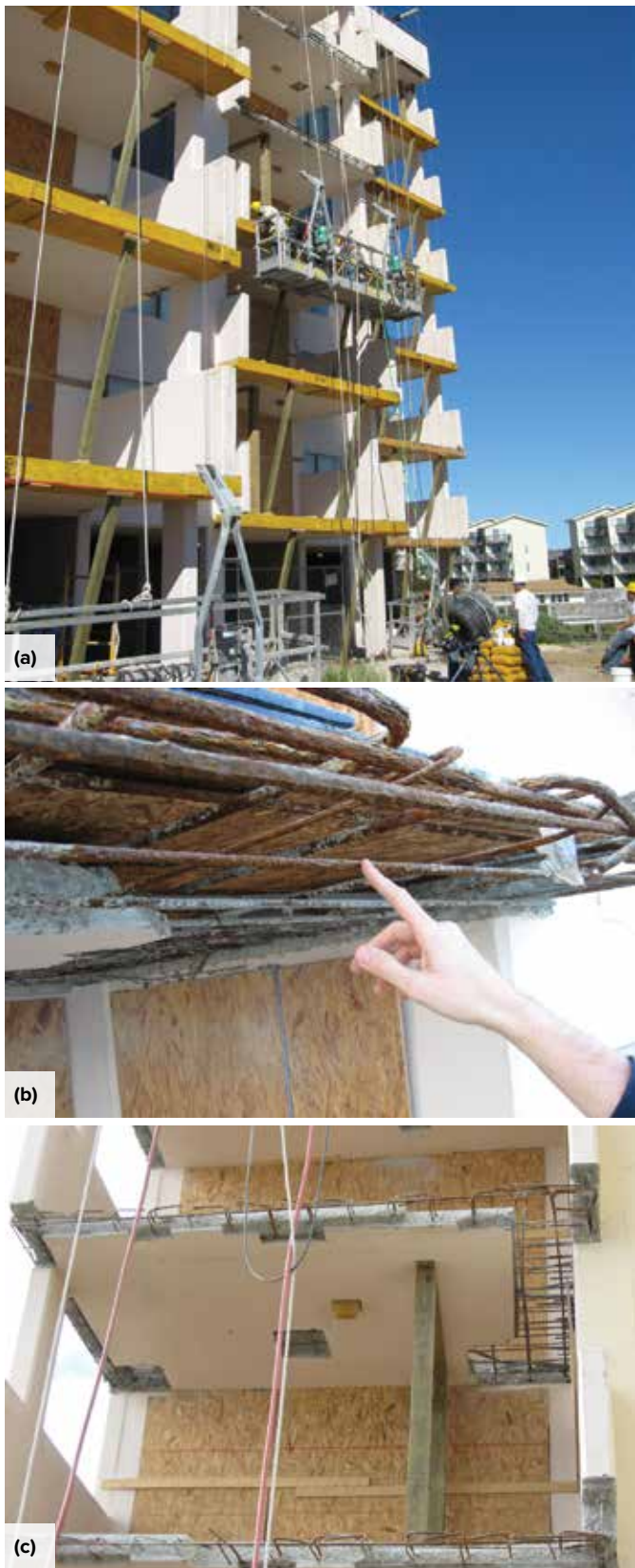
Fig. 4: Balcony repairs: (a) general construction access with visible swing stage; (b) extent of distress; and (c) one of the more severely distressed balconies requiring shoring. Note demising walls at balcony sliding glass doors
