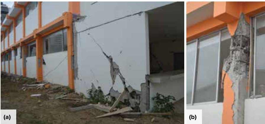
Fig. 5: Damage caused in two buildings by the 2016 Ecuador Earthquake: (a) shear failures in masonry infill walls; and (b) shear failure in a short, ground-level column above infill walls (after Reference 23, licensed under CC BY-SA 3.0)
