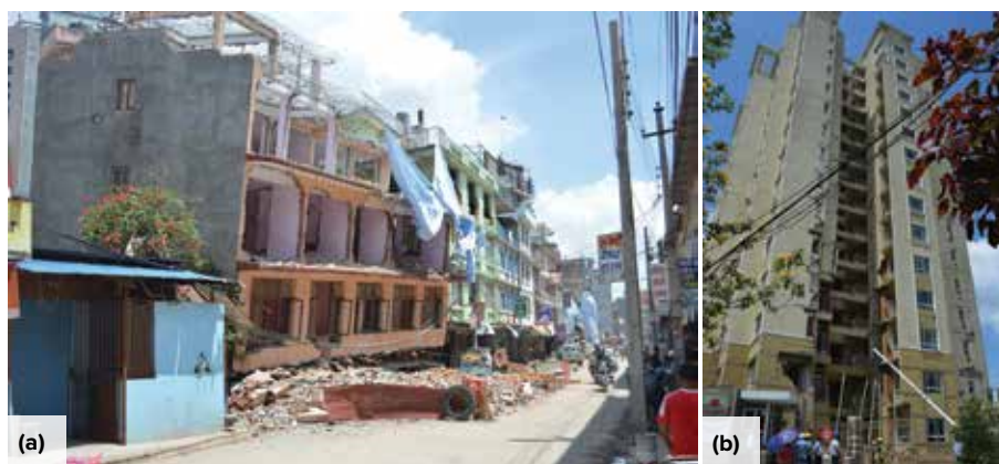
Fig. 3: Buildings damaged in the 2015 Nepal Earthquake: (a) low-rise building (after Reference 18, licensed under CC BY-SA 3.0); and (b) high-rise building (after Reference 19, licensed under CC BY-SA 3.0)
