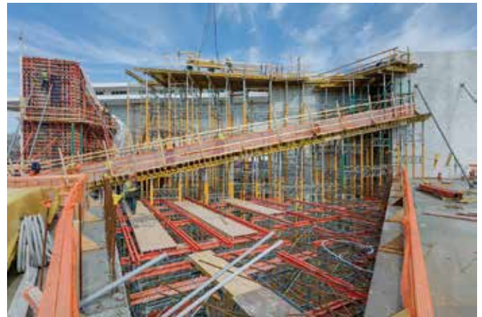
Fig. 5: Shoring and formwork at the Welcome Pavilion. In the background, 40 ft (12 m) tall shoring is in place for the elevated roof slab that forms the upper atrium ceiling. In the center of the image, variable-height shoring was erected for the 92 ft (28 m) long post-tensioned concrete beam needed to support the vaulted slab that forms a lower ceiling in the pavilion. The contour of the vaulted slab was formed on boxouts fabricated using a CNC router. The boxouts were supported by the orange deck members in the foreground
