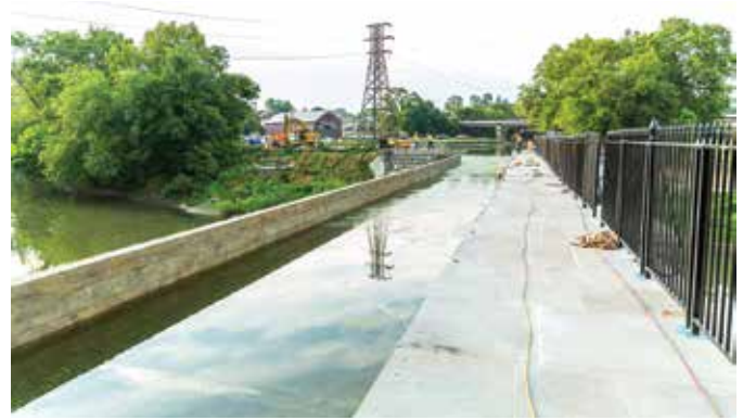
A view from the towpath side of the aqueduct, showing the interior of the concrete wall that was stamped and stained to resemble wood
